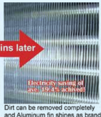
Air heat exchanger is stuck by the greased dirt.
