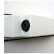
Cable entry with rubber grommet.
