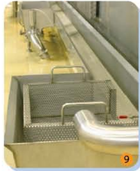
Recirculation type CIP system
