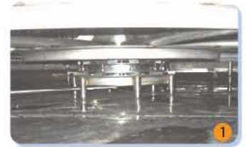
Bottom main bearing of Spiral drum
