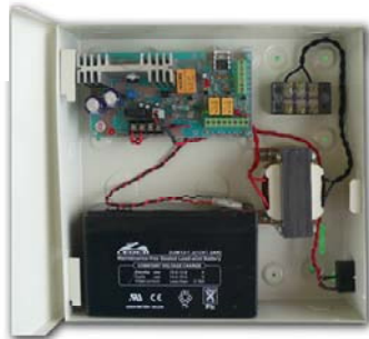
Power Supply & DC UPS
